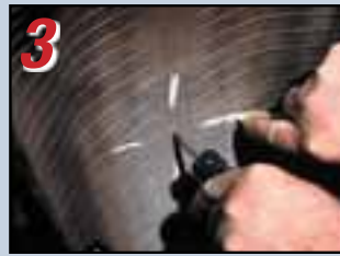
3 Inspect the damage using a 190 awl, determine if one-piece or two-piece repair is required.
